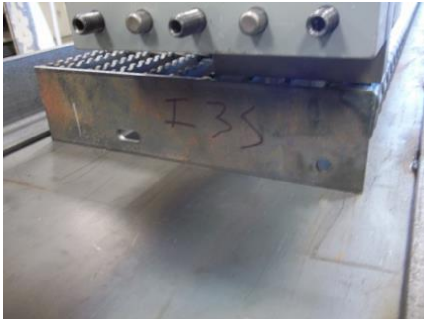
Photo No. 10 Part 3 - 29 CFR 1910.24(c) Loading Shear
