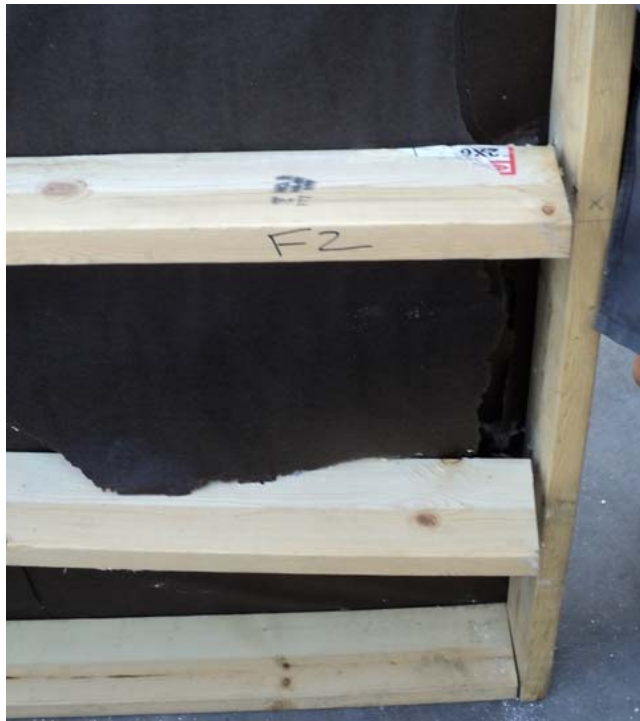
Photo 5 – Typical Failure (F2)
