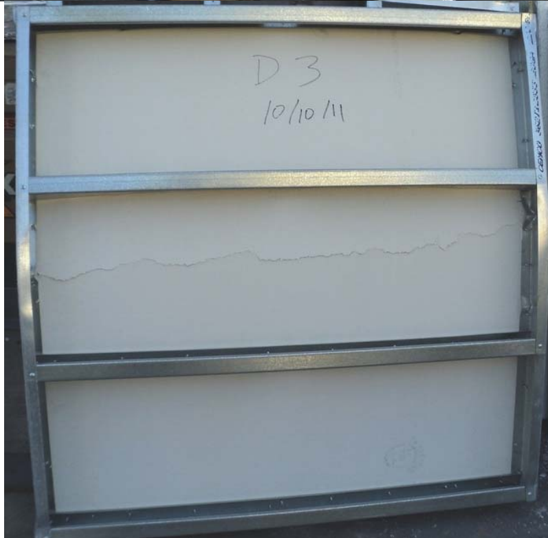
Photo 3 – Typical Failure (D3)
